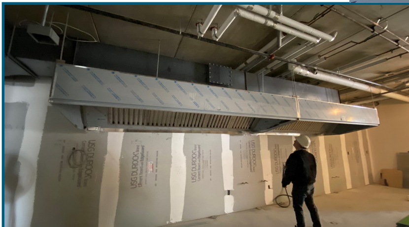
Kitchen hood is installed.
